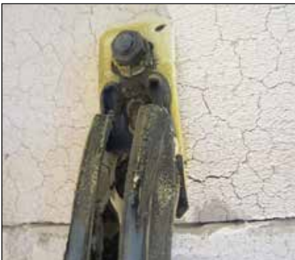
MQK bracket after the fire test, partial tearing away of the channel from the base plate
