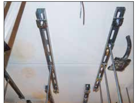
Directly-installed channel with single load
