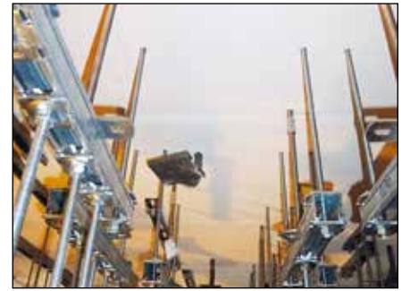
MQ-41, suspended installation, MQA installed on the underside
