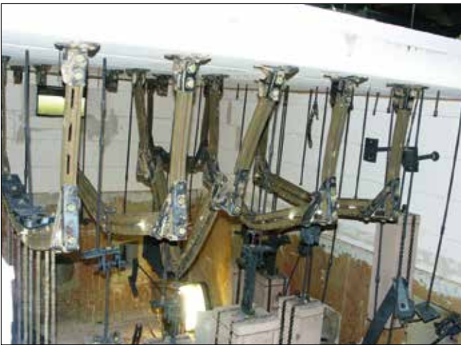
U-support with single and multiple load after the fire test
