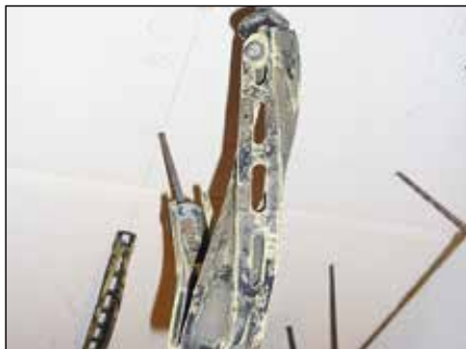
MM-C-45 channel, suspended, with single load after the fire test
