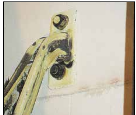
MQK bracket after the fire test, severely deformed
