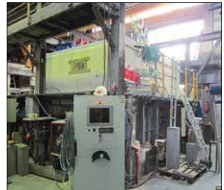
Furnace: The upper section is built for each test out of gas concrete blocks
